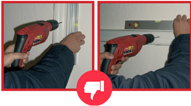
Duct installation without built-in level
