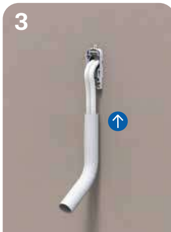
Place the refrigeration pipes and the power supply in the corrugated protection pipe
