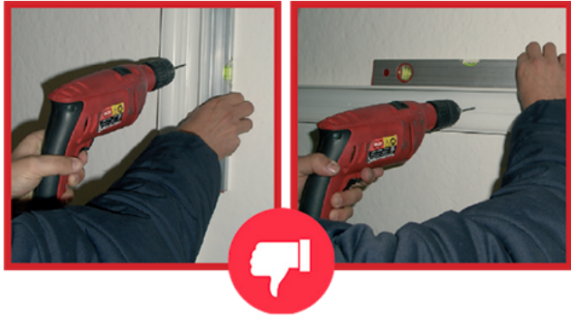
Duct installation without built-in level
