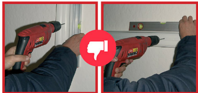
Duct installation without built-in level
